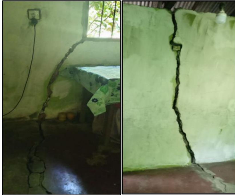
Figure 2: Cracks in the wall and floor of the house
