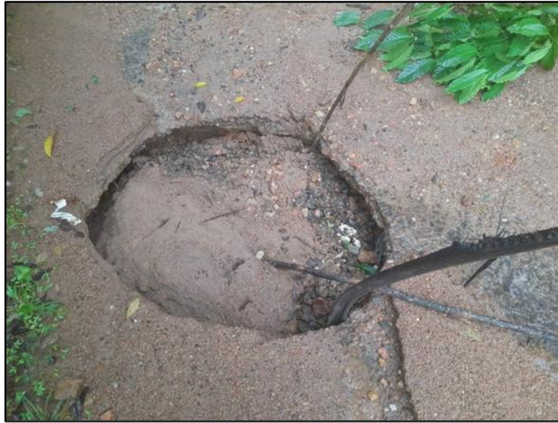
Figure 3: Fractures on Slopes
